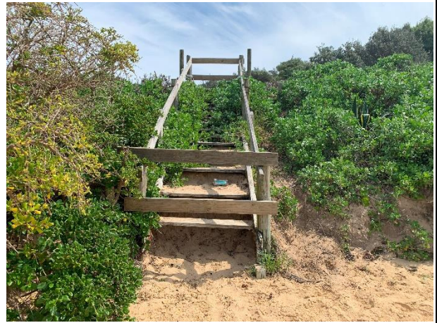
Plate 4. Existing staircase in disrepair on the foredune
