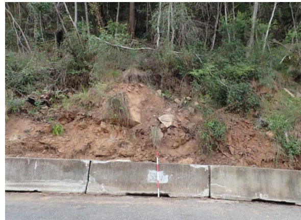
Plate 2. View to north. Settlers Road. Fresh landslide material in lower five metres, with more consolidated colluvium higher up, covered in native vegetation. Landslide material included large angular sandstone boulders, shale, clay and sandy soil.
