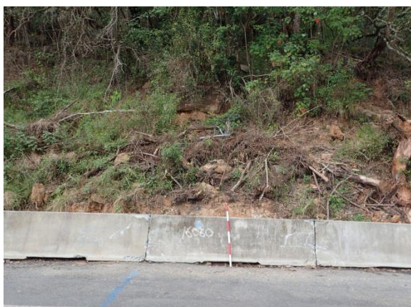
Plate 3. View to north. Settlers Road. Lower landslide material near roadway, with vegetated consolidated colluvium on higher slopes.
