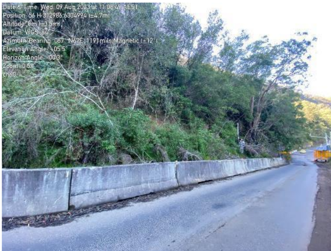
Figure 3-3 Views of the landslide looking east
